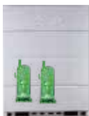
Intelligent load-bearing between compressors during normal operation
